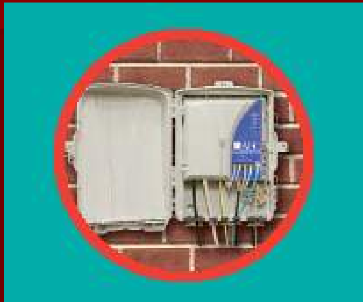
Optical Network Terminal (ONT)
